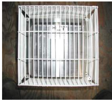
VIEW OF SAFETY CAGE
